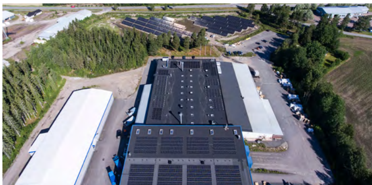
Solar park and solar installation on the roof at Coreplast Laitila Oy.
