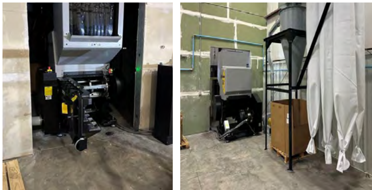
Plastic grinder at Gibo Inc. installed in a newly established area in the factory.
